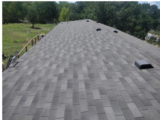
Picture-Perfect is the only way to describe this beautiful work of art that Double SS Construction constructed with roofing materials donated by Ja-Mar Roofing of Buda, Texas.
