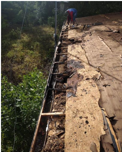
After tearing off the old roof, it was evident Edie's roof was in desperate need of a makeover.
